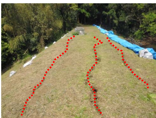
Photo 5. Cracks of reservoir (Ohzu)
