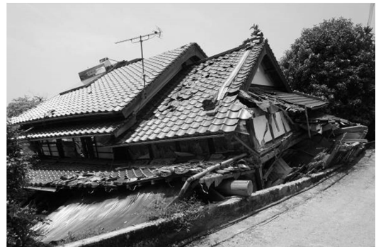
Fig.1. The damages of fine wooden farmhouses.
