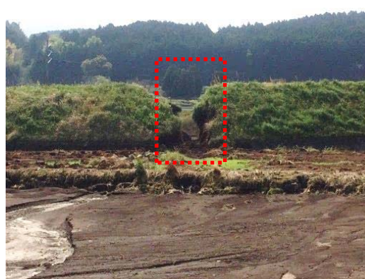
Photo 5. Collapse of reservoir (Nishihara)
