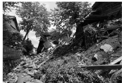
Fig.3. The serious damages of retaining walls.
