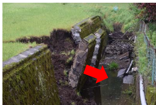
Photo 4. Fall-down of paddy wall
